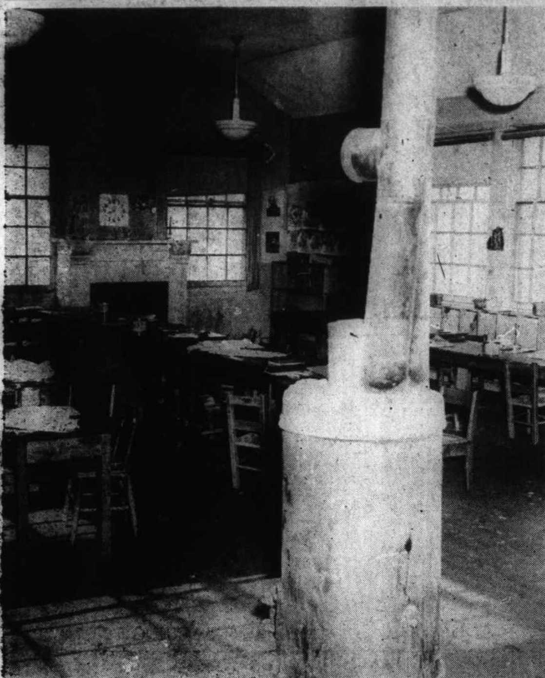
An interior view of one of the poorly constructed rooms at Hiwassee Dam School, shows that some of the rooms are still heated with pot-bellied stoves. The school is a building originally built to be used as a dormitory for TVA workers during
