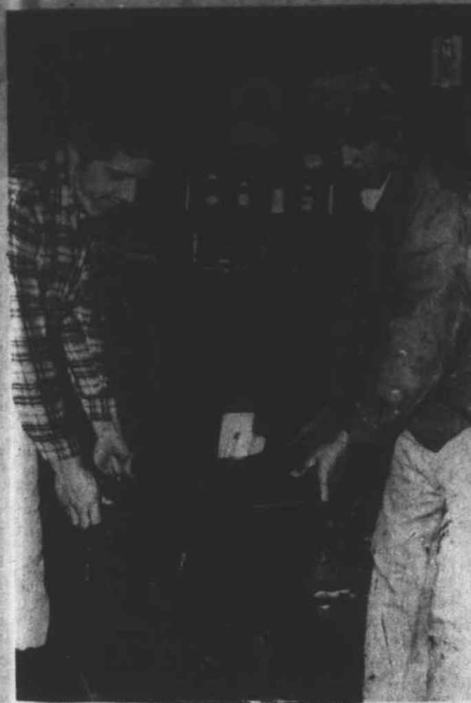
ANA's Home Repair Crew is shown installing new heater. In background can be seen fireplace that has caught on fire twice.
