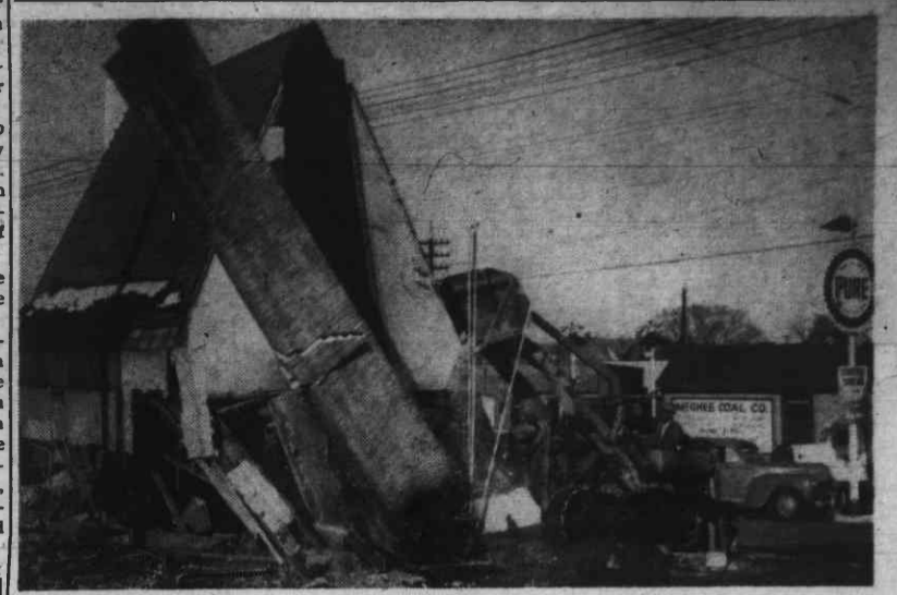
Pictured above is the demolishing of the old Speight's Auto Service Station to make room for a new and modern Pure Oil Station to be located on the same spot at the corner of Fayetteville and Pettigrew Streets. The new establishment is fast becoming a reality with the builders now putting on the finishing touch. Plans for a Grand Opening will be announced in this newspaper during the early part of March.
