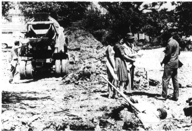
CONSTRUCTION OF THE NEW $150,000.00 M. Rebecca Stith Memorial Hall gets underway at Southeastern Business College in Durham. Shown looking over plans are (L to R) Miss Lois Cunningham of Gladys, Virginia, President of the House Council; Mrs. Lorraine Stith, Dean of Southeastern; D. W. Stith, President of SBC and Rev. L. E. Hunt, member of the Board of Trustees. (Photo by Purefoy)
