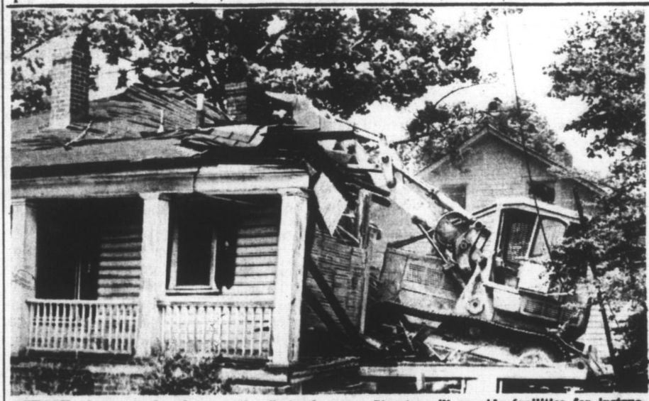
ATTACK—A top loader devours the first of four houses which fell this week on the site of North Carolina Central University's planned Communications Building. The $2.2 million building, at the corner of Fayetteville and Law-
