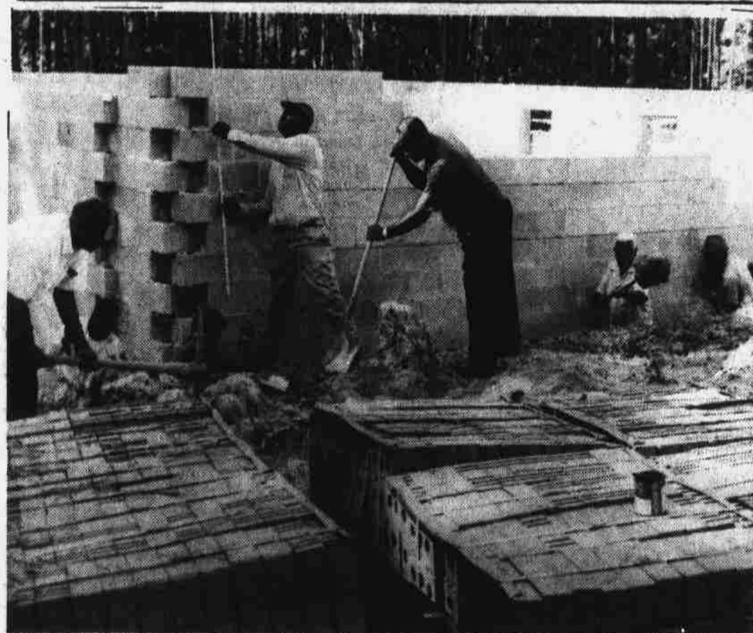
PRINCE HALL MASONIC TEMPLE UNDER CONSTRUCTION ON 301 COOK ROAD — Some members of Doric Lodge No. 28 Free and Accepted Masons, Prince Hall Affiliation are shown working on New Masonic Temple being built on Cook Road. From left to right are Emmett Martin, Odell Fields, John Tucker, Frank Jacobs, Sr., Otis M. Thorpe, Jr., Edgar Alston and James Henry.
