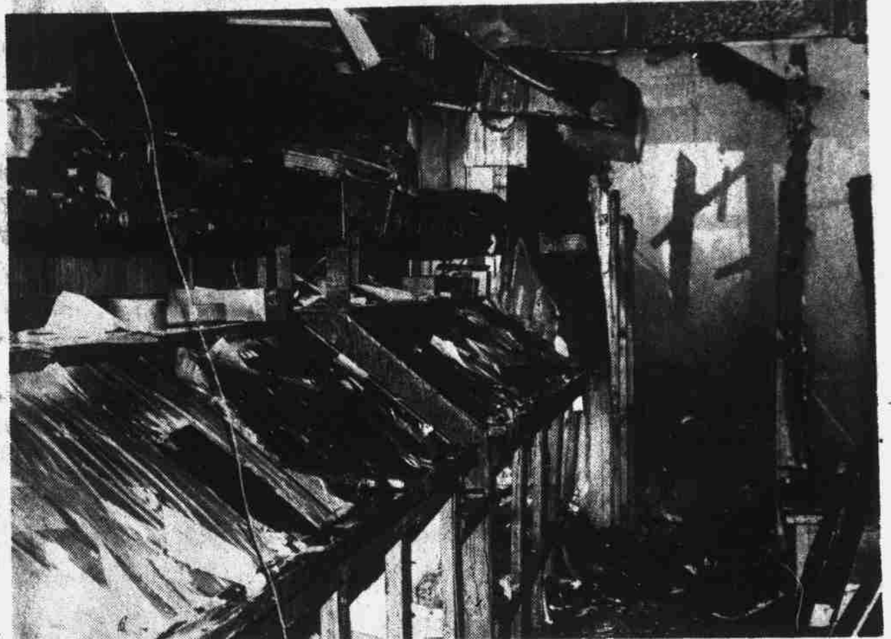
COPY AND MAKE-UP ROOM in shambles, beyond which the second and third floors had collapsed on mailing and typesetting rooms. (Photo by Kelvin A. Bell)
