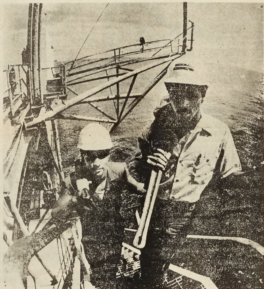
College students Norman Spruill (left) and Gregory Twyman traded in textbooks for pipe wrenches to learn more about the petroleum industry during summer training at an Aminoil offshore oil production platform.
