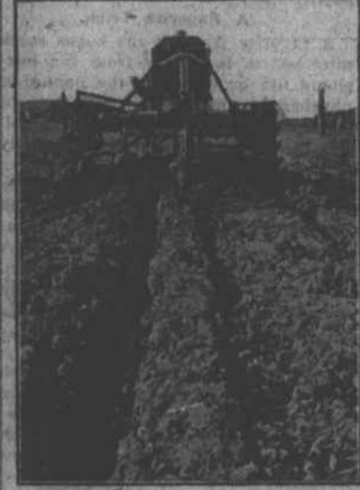
A Modern Machine Working on a Rutty Highway.
