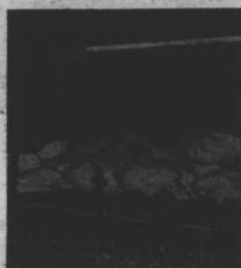
An installation of Westinghouse sterilamps in a poultry house at New Hope, Pa., fights poultry infections and improves vigor and health of hens while they sleep.
