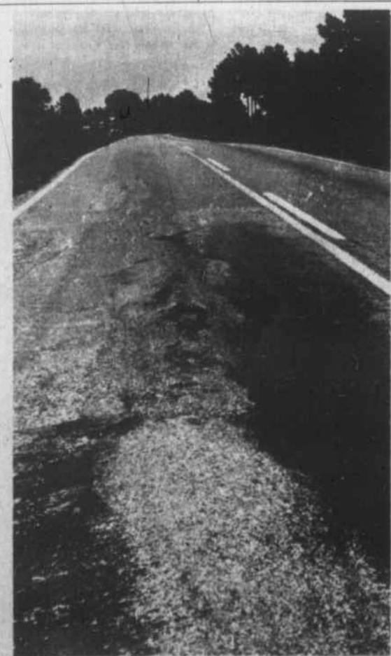
This Is A Hole In N. C. 56
