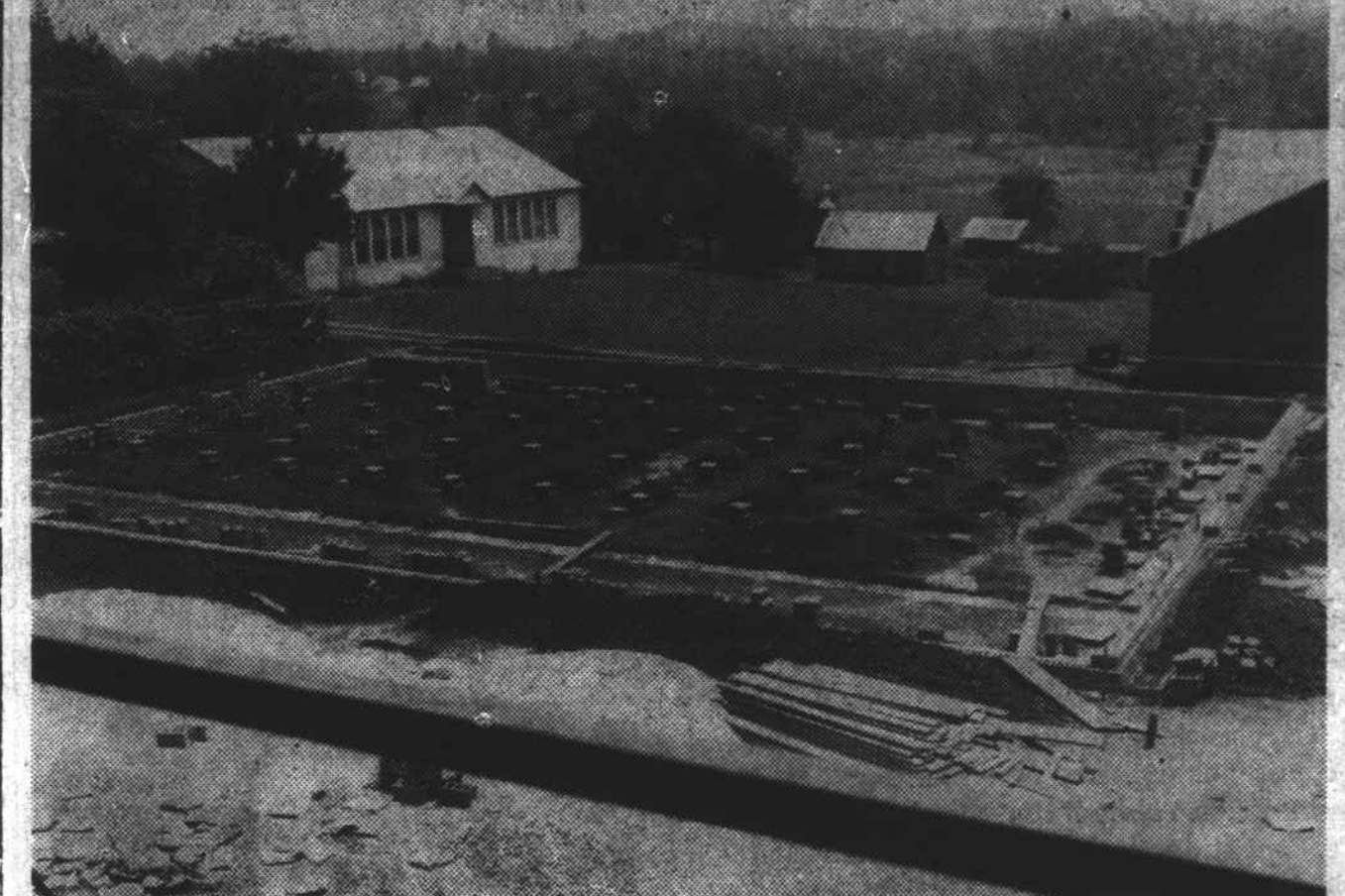
Work has begun on construction of the gymnasium for Wilkesboro school and efforts will be made to complete the structure in time for use in the basketball season. Jesse Walsh, of Wilkesboro, is construction foreman, with the work progressing under direction of the building committee, of which Joe H. Pearson is chairman, and school officials. The gymnasium, located on the school property in the rear of the high school building, will be 75 by 98 feet and will be built of blocks, wood and steel. Space is being provided for about 1,000 spectators. A building fund of $12,000 was made up of contributions and by school activities.—(Photo by Lane Atkinson, Jr.)
