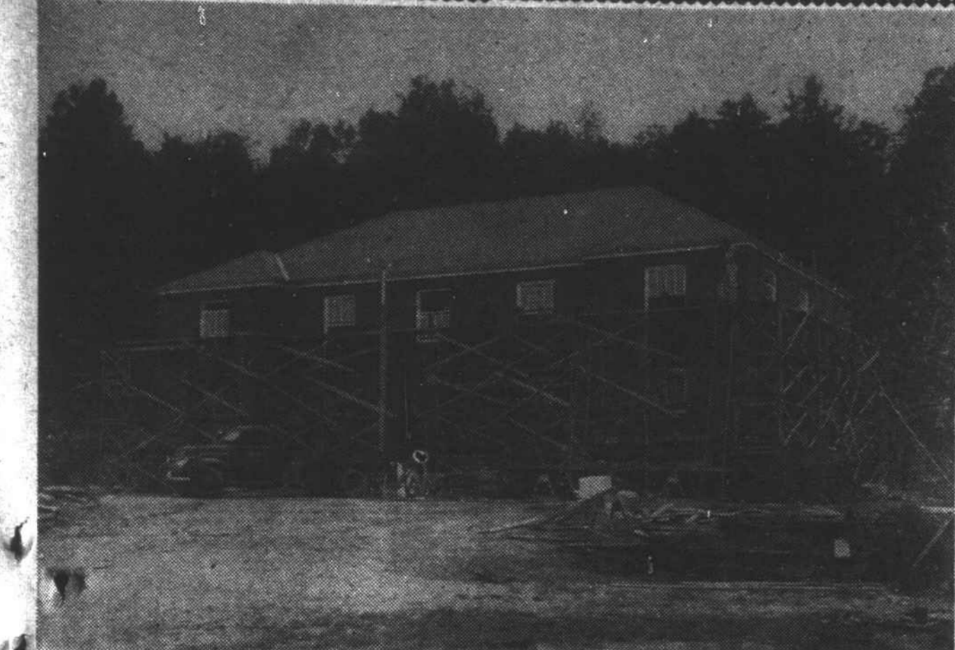
This photo shows work in progress on construction of the new Eighth Division offices of the State Highway and Public Works commission. Previously shifted from town to town in rented quarters, the eighth division office will be permanently located in the new brick veneer building, which is being erected on State Highway property adjacent to the prison camp and highway division garage just outside of this city on highway 115. The new building, which will be ready for occupancy in the near future, will have nine offices, assembly room and modern conveniences.—(Photo by Lane Atkinson, Jr.)
