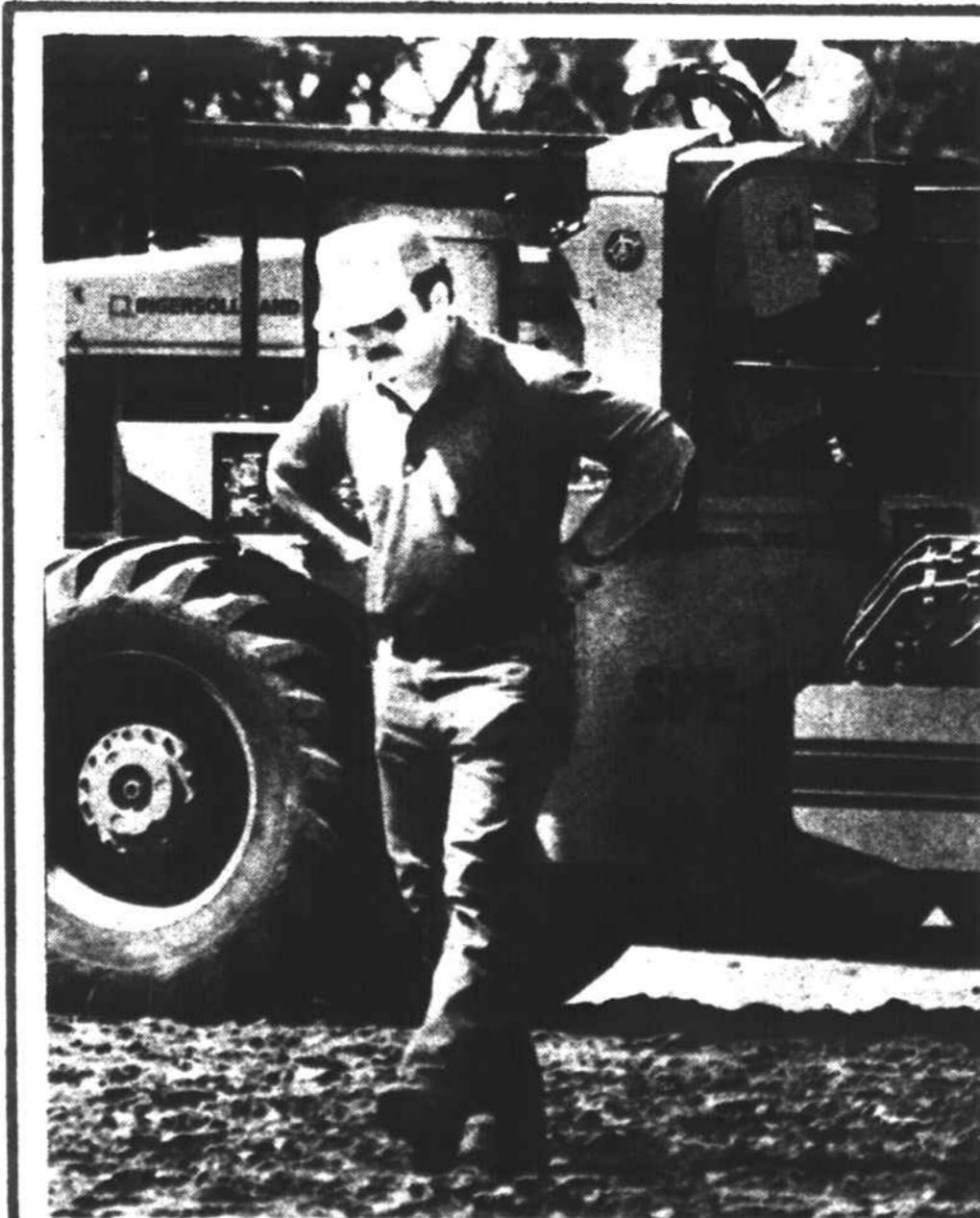
Low black participation: Workers on the site of the convention center expansion (photo by James Parker).
