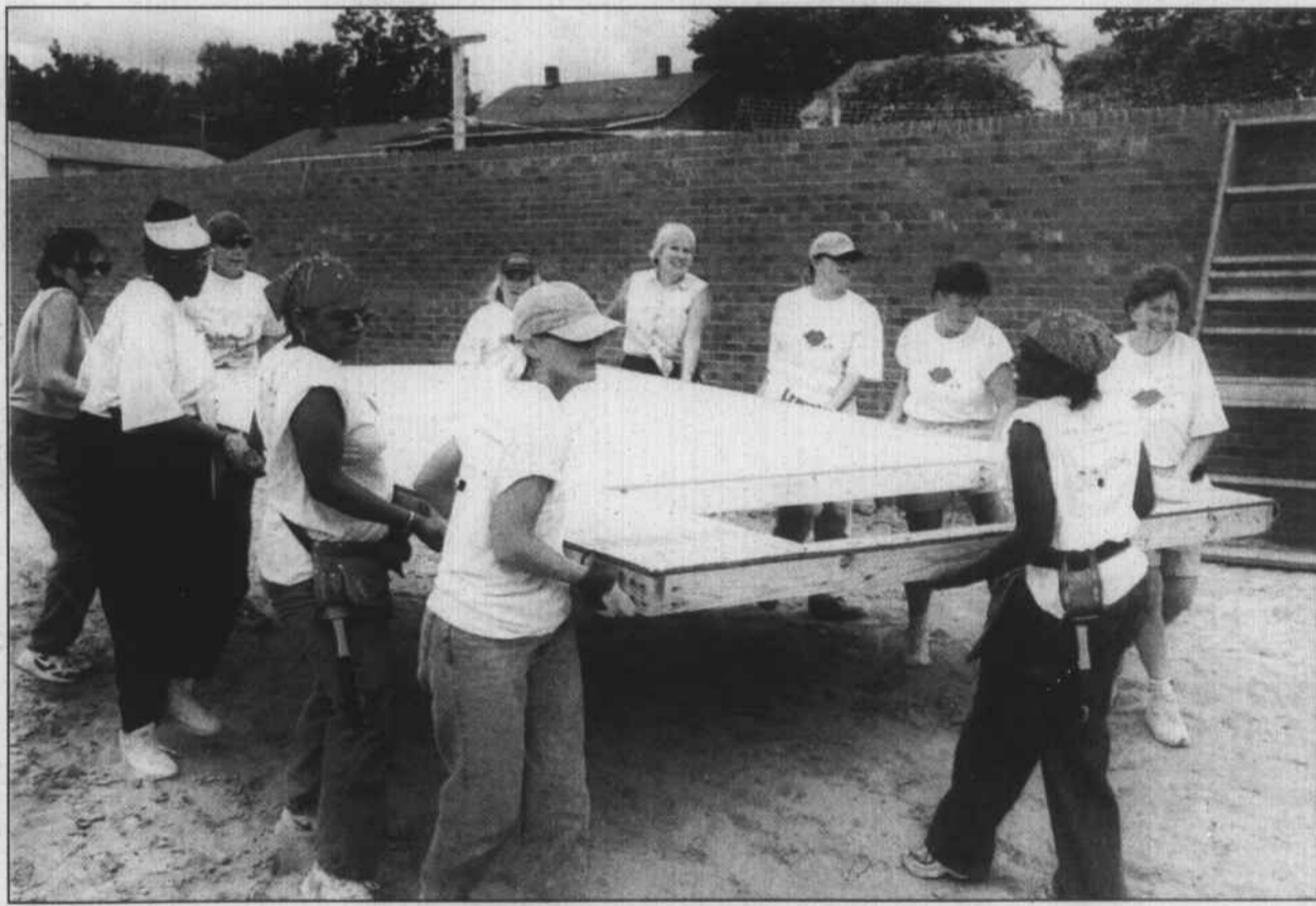
Local women continued a Labor Day tradition last weekend, partaking in an all-female build for Habitat for Humanity of Forsyth County. Women from local companies such as RJR, GMAC and Sara Lee gave up their holiday to haul and hammer at a site in Neil's Place off University Parkway, where people of both genders were busily working on other homes as well. The all-female house should be completed by year's end, and a local family will move in soon after it is completed.
