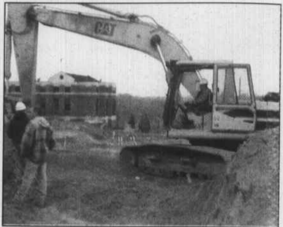
Workers clear space on the west side of Martin Luther King Drive to construct the new dorm, Rams Commons.
