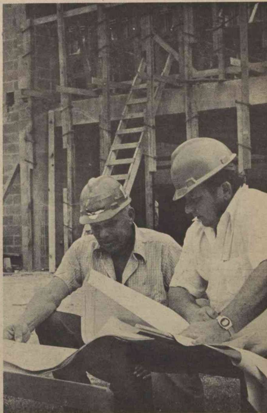
Job superintendent Durwood Sauls, right, and Russell Trogdon, both of King Hunter Construction Co., study architect's plans for construction of the new gymnasium-physical education center. The facility is now about two-thirds completed.
