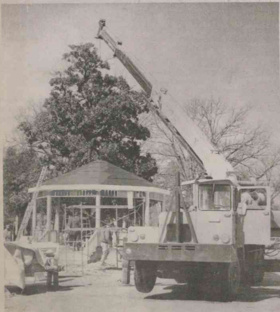
A large crane was required to remove the college bell from atop McDowell Columns and lift into place in the gazebo.
