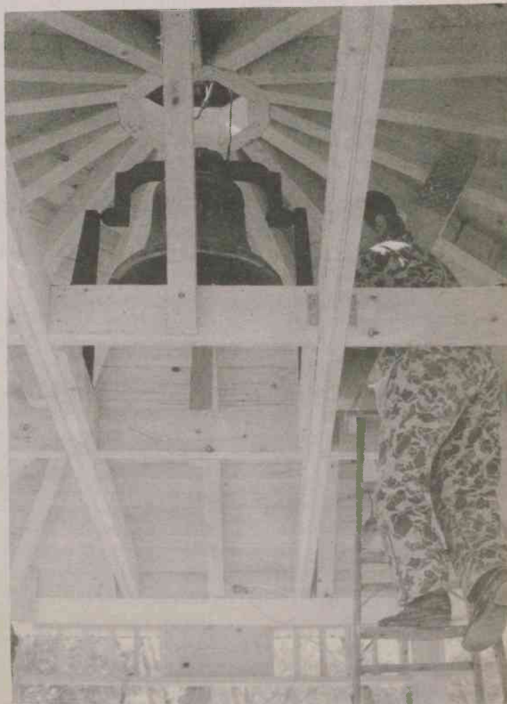
A member of the maintenance department secures the bell in the brackets. Heavy, braced joists were necessary to carry the weight of the historic bell, which will be rung on special occasions.
