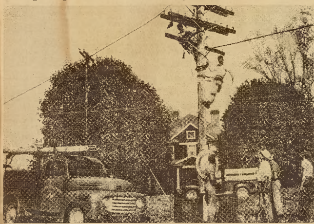
Work has been started on the installation of the telephone cable from Brevard to Rosman and the line and the Rosman exchange are expected to be in operation during '53. Inter-toll dialing will be used for the Rosman exchange, and there will be no charge for calls to and from Brevard and Rosman. Uppermost in the picture on the telephone pole is Lawton Houston and Erwin Holden can be noted catching a piece of equipment being thrown up from the ground crew. From left to right on the ground are: John Hoover, Max Wilson, plant superintendent, Charles Pickelsimer, Jr., and Carroll Merrill. (Times Staff Photo)
