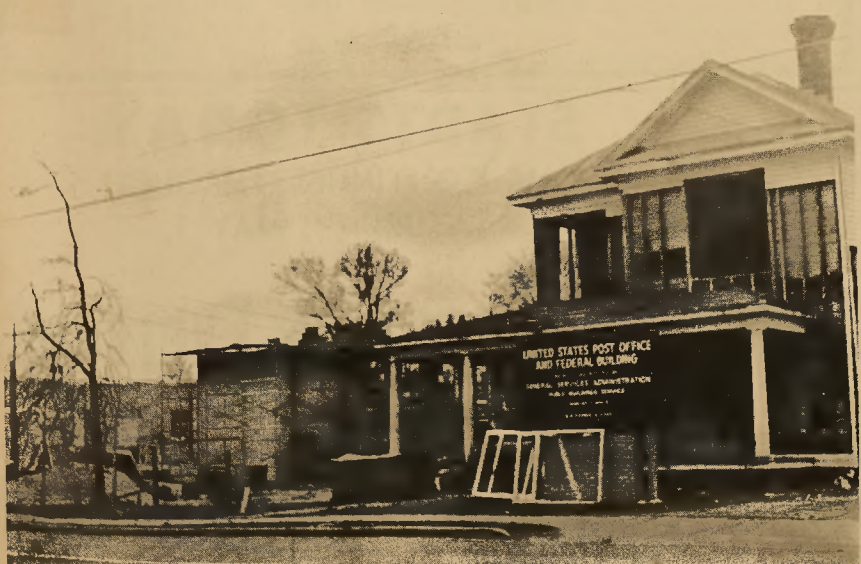
PROGRESS IN ACTION — Walls fall in the foreground and walls rise in the background and the new post office building begins to take shape in Rich Square. The old Kate Stephenson house is being torn down to make way for needed space to complete the
