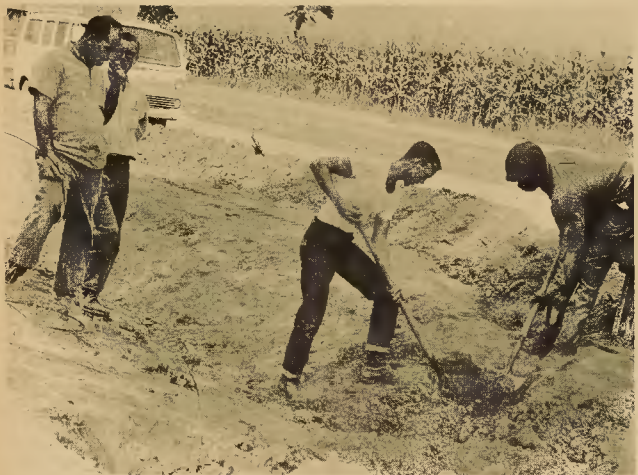
BURIED CABLE—Telephone Plowing Co. crew digs out a telephone line along the road near Northampton County High School to restore service after state highway crews widening and resurfacing the road finally redigging the ditches. This scene in front of Mrs. Carrie Johnson's house on Route 2, Conway, was repeated a number of places along the road. Telephone lines in the area are buried and redigging the
