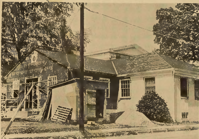
ADDITIONAL SPACE —The construction of additional office space in the county agriculture building will provide adequate space in Jackson for all county agricultural extension personnel. Expected to be ready for occupancy by January 1, the total cost of construction will be around $15,000, including $1,500 for a new heating system and roof for the entire building.
