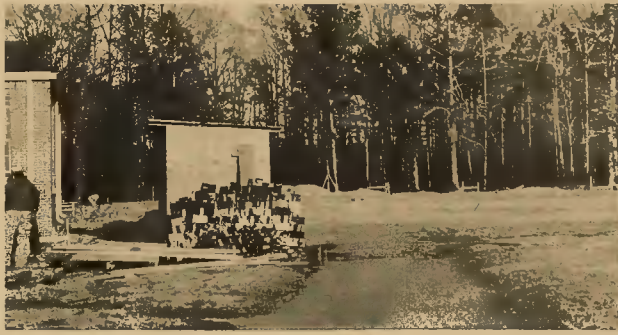
EXPANSION BEGINS at Talon, Inc., Woodland, with clearing of land at rear of the present plant for addition of a new raw material warehouse. Construction markers at the edge of the woods show the size of the zipper plant's second expansion since opening here in 1953. Upon completion, the new construction will free existing warehouse space for manufacturing operations.
