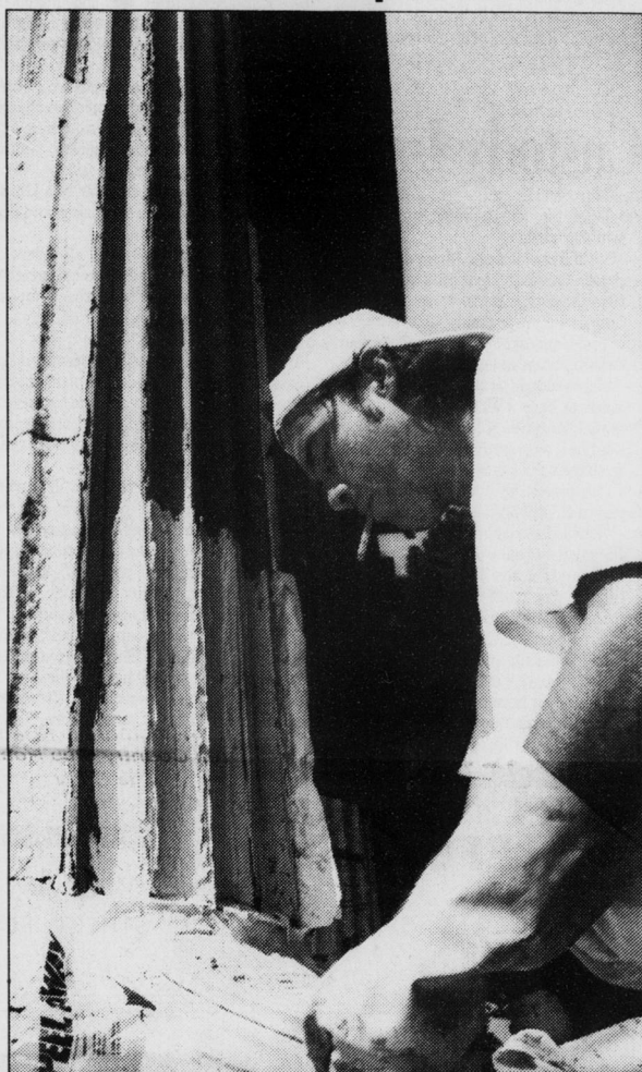
Jeff Arndt of Maynor and Hennessey Construction patches the Playmakers Theatre columns Thursday afternoon as part of Bicentennial restorations.
