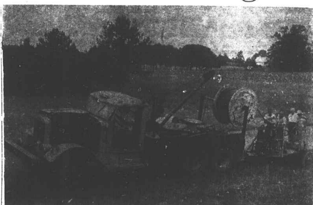
GOES UNDERGROUND — A crew is shown burying telephone line for Carolina Telephone and Telegraph Company in front of the Osborne Limer home at Afton on Tuesday morning. (Staff Photo)
