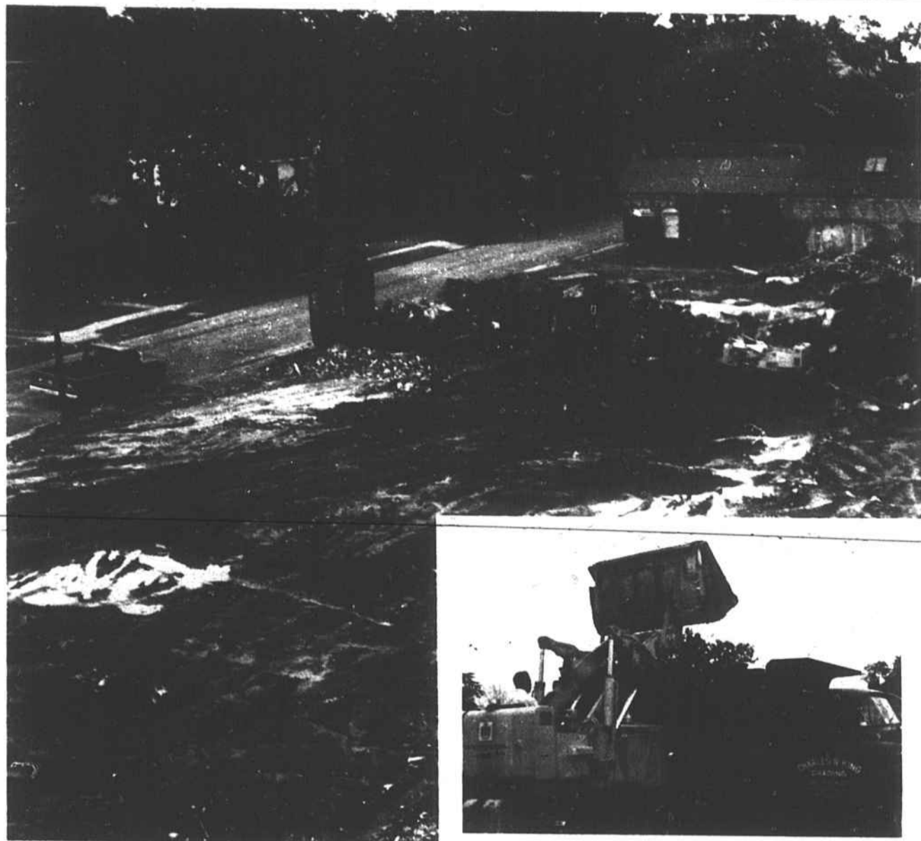
Scott Gardner, manager of Warrenton Furniture Exchange, said yesterday that he hoped that removal of debris from the warehouse fire last Tuesday would be completed this week. Pictured are workmen removing debris.
