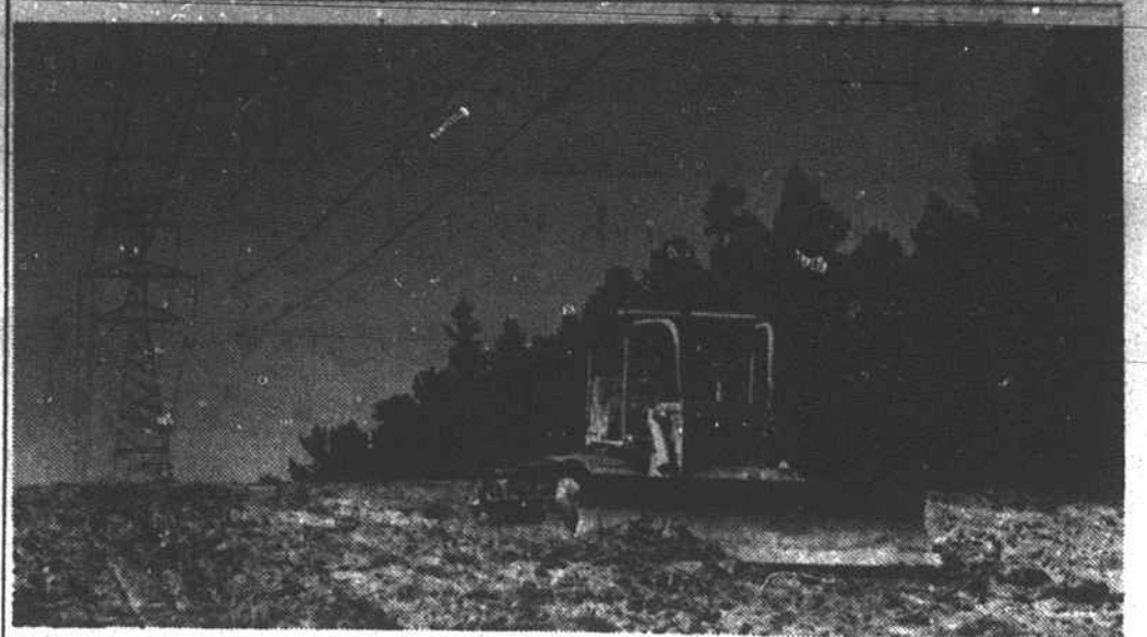
POWER PLUS—Preparing the land for future seeding, a bulldozer moves beneath Carolina Power & Light Company transmission lines. CP&L's program of helping develop the right-of-way land into either a wildlife area or farmland was the first in the Carolinas and a model project for the nation's electric companies.
