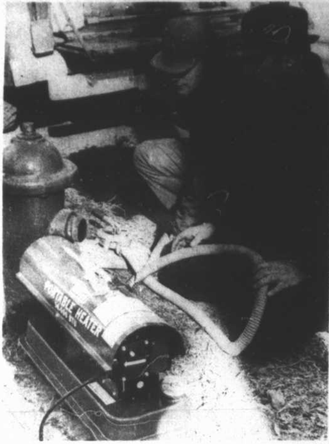
Bill Neal, right, and Jimmy Ross of the Warrenton Water Department apply a heater to a frozen fire hydrant. Freezing pipes have plagued both commercial and residential users in Warrenton during the month of January. Only isolated inconvenience has been caused water customers in Norlina, town officials reported this week. [Staff Photo]
