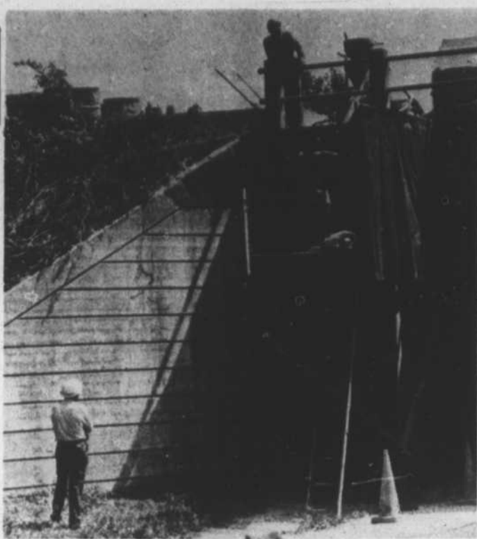
UNDERPASS FACELIFT —A railroad bridge repair crew is shown Monday beginning renovation of the underpass on U. S. 158 and 401 in Norlina. Cracks are being repaired and leaks patched during the operation. One-lane traffic is required while the work is in progress. (Staff Photo)
