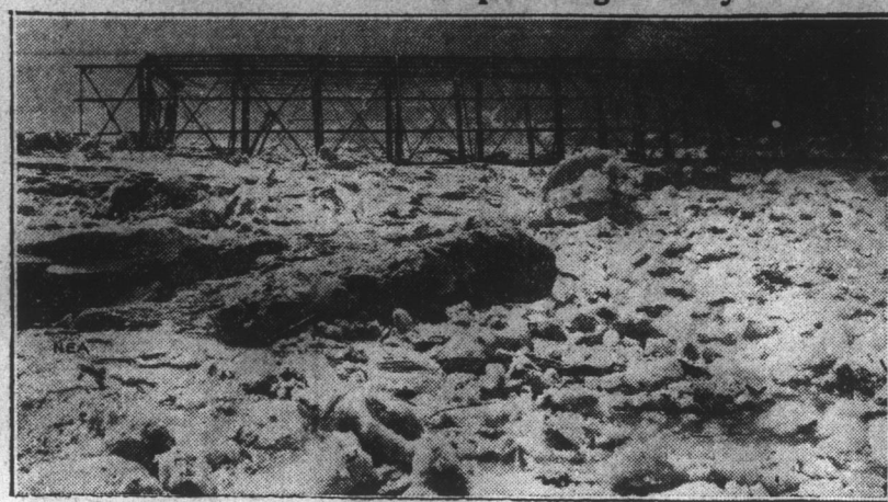
Thousands of tons of ice borne downstream by the flooded Alleghany river at Franklin, Pa., exerted such tremendous pressure that a steel bridge was broken in half and part of it swept away. The picture shows two spans of the bridge lodged, upright, in set upright by the pressure.
