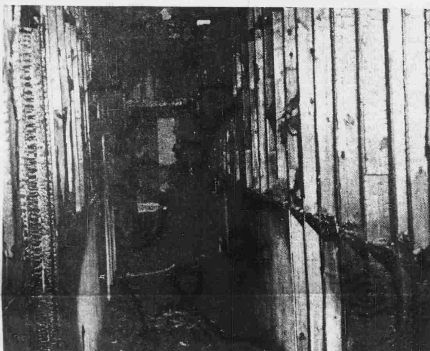
SWAIN DAMAGE —Gutted by fire Thursday night, this corridor of Swain Hall stands charred and practically destroyed after flames ripped through the building. Damage to the building—which housed the radio and television studios—was estimated to be around $60,000. (Glenn May Photo)
