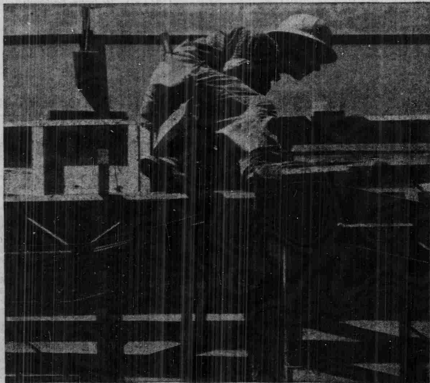
CARPENTER AT WORK—Here is a workman finishing the last stages of the new language building. He is building the wooden molds for the concrete beams that support the building. Looks as if he's caught his legs between the board and the concrete!
