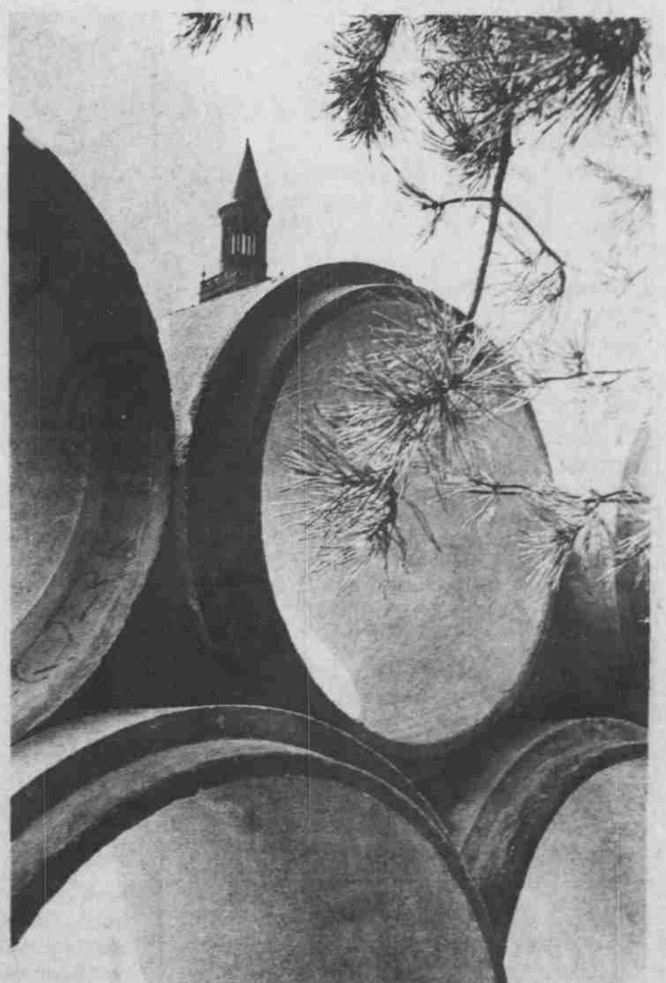
BEAUTY OUT OF THE mammoth destruction — down by the Wilson library, new drainage pipes for the proposed undergrad library lie stacked on top of one another. The modern wings on the library will be completed by the Fall of 1968.
