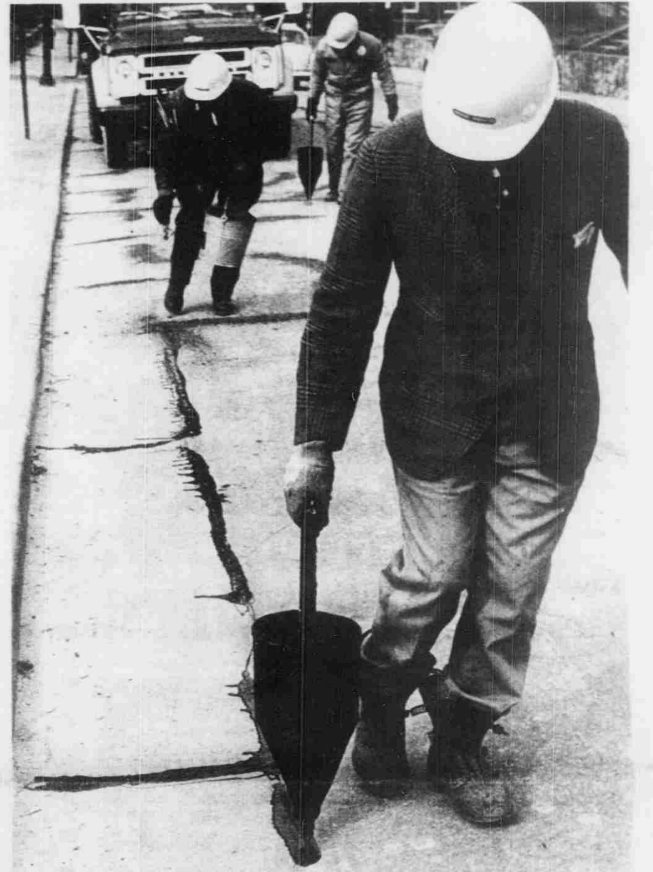
Workers were busy this week filling in cracks in the pavement on Hillsborough Street with tar to prevent damage from water drainage. The street may be repaved this summer, according to Chapel Hill officials. (Staff photo by Johnny Lindahl)
