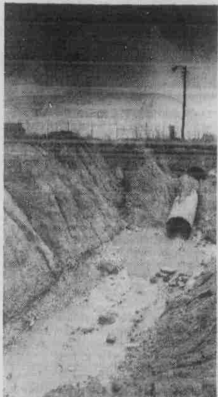
Runoff pours from drainage pipe at Shearon Harris construction site.
