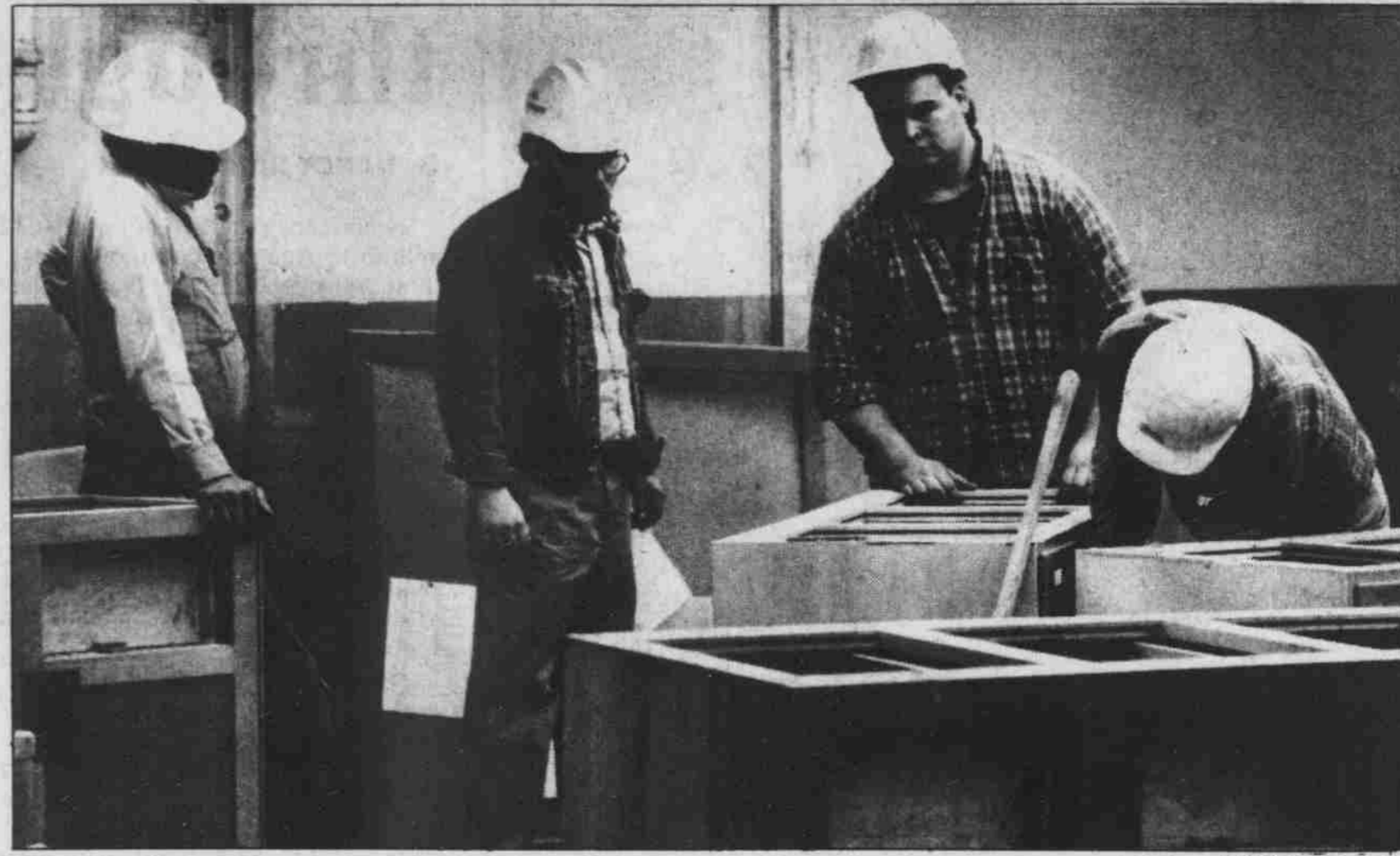
Construction workers at the new joint Glaxo-UNC laboratory in Venable Hall DTH/Tony Deifel
