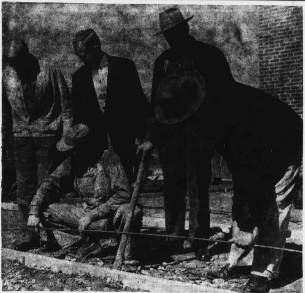
SIDEWALKS FOR THE NEW Franklin High gymnasium sent the Macon Board of Education outside after its business meeting Monday morning. The board is shown talking over the project with contractor Wiley Clark (kneeling)—(L to R) Chairman Erwin Patton, Supt. Holland McSwain, George Gibson, and C. C. Sutton.
