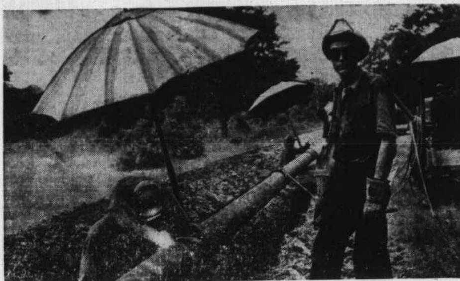
Because it is 99 in the shade not counting the heat from the arc, welders on the pipeline that is being rushed to feed the oil-starved eastern seaboard are given some relief by the sunshades. The men work in pairs, one at each end of a pipe section. This particular line is made up of partially used pipe-line systems which were dug up and relaid in directions that will accelerate the flow of oil to the Atlantic seaboard from the oil fields of the southwest. (Central Press)
