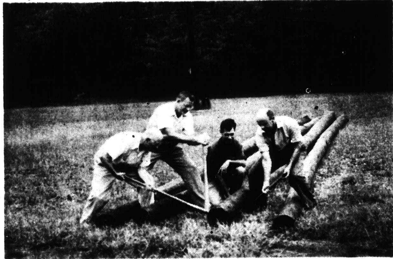
Shown above, left to right, Lions John Corbin, Mack Deitz, Mike Strong and Dennis Barkley as work was begun on the new lighting system for Mark Watson Field. The new lights are now completely installed and ready for the opener with Hayesville tomorrow night at 8:00 p.m.
