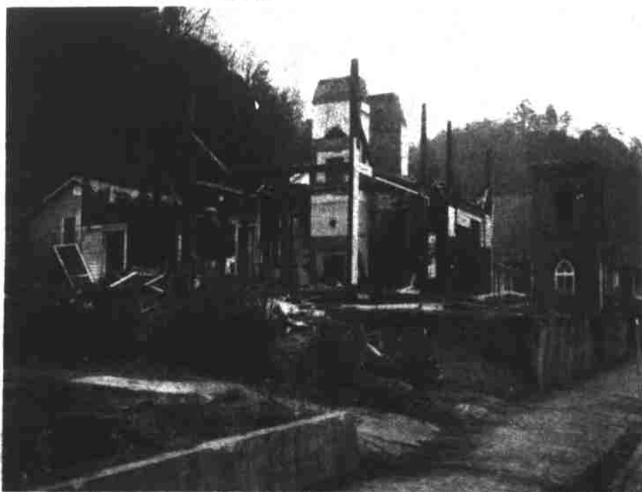
ANOTHER LANDMARK IN MARSHALL is being torn down in preparation of building low-rent housing units. Picture above shows the remains of the "Old Tom Ramsey Place" located near the United Methodist Church on Main Street. In all, four separate sites in Marshall have been secured for the 50 units planned.
