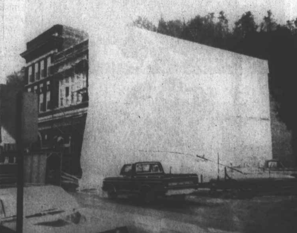
PLASTIC WALL, beside the First Union Bank protects the workmen regardless of the weather, as they remodel the structure on
