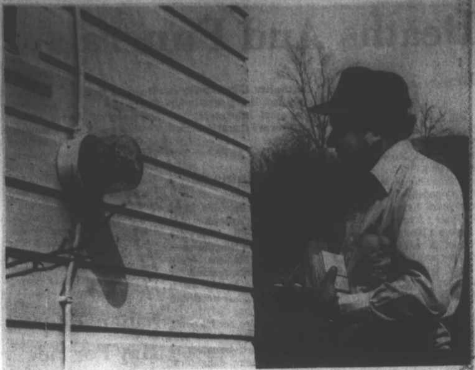
RONNIE RAY makes one of his six-month checks of an electric meter along the Doe Branch route in Madison County backcountry.
