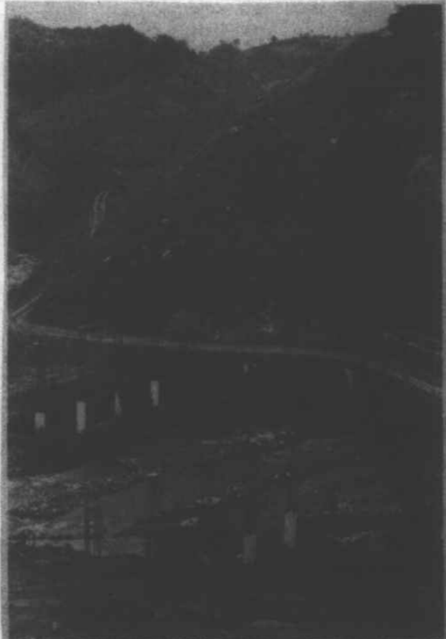
A $1 MILLION bridge will span the Ivy River here, and 1.6 million cubic yards of the hill beyond will be removed.
