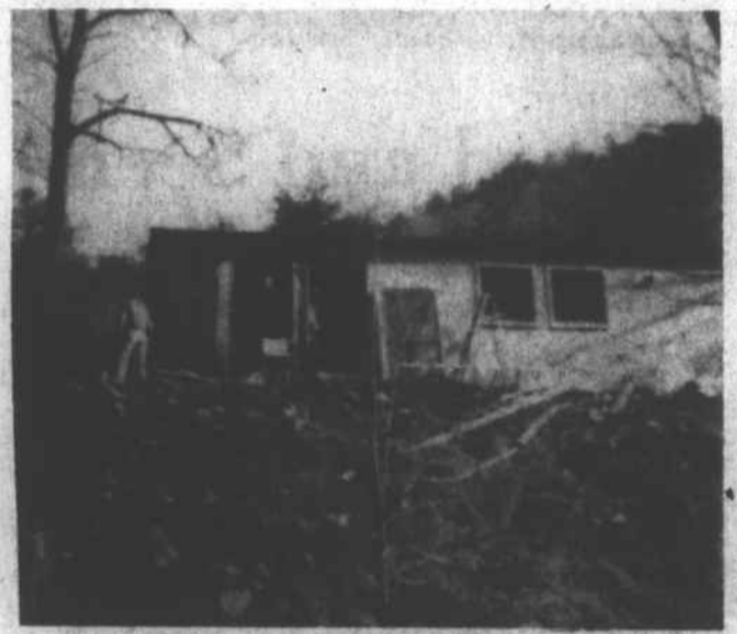
THE HOME OF JESSIE AIKENS on Spring Creek Road was photographed before the rehabilitation work began.
