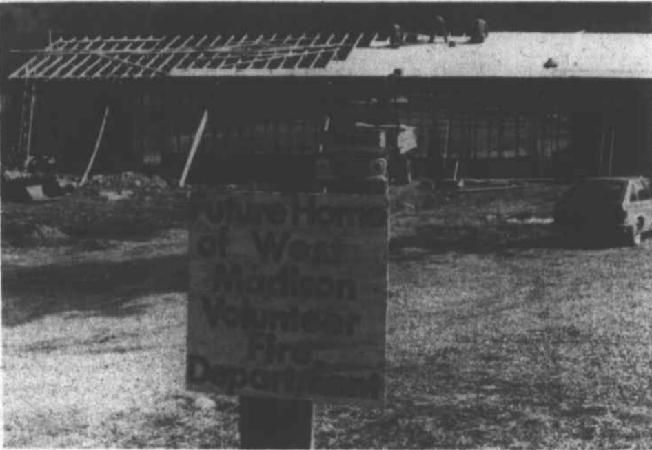
THE WEST MADISON FIRE DEPARTMENT building is beginning to take shape. Volunteers from the community are shown working on the roof to the new headquarters. Men and women
