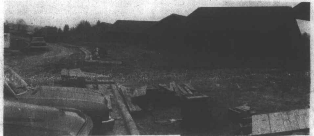
WORK IS NEARLY COMPLETED on new 40-unit housing being constructed in Mars Hill by the Madison County Housing Authority. The two
