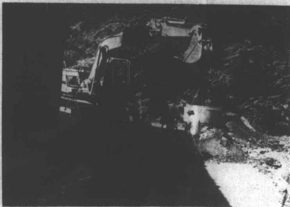
WORKMEN CONTINUED EXCAVATION ON HILL ST. IN MARSHALL THIS WEEK after engineers recommended route over possible alternative that would have required digging behind the county Court House.
