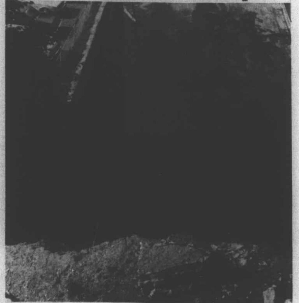
TEN-FOOT SECTION OF HILL STREET COLLAPSED following heavy rains Sunday.
