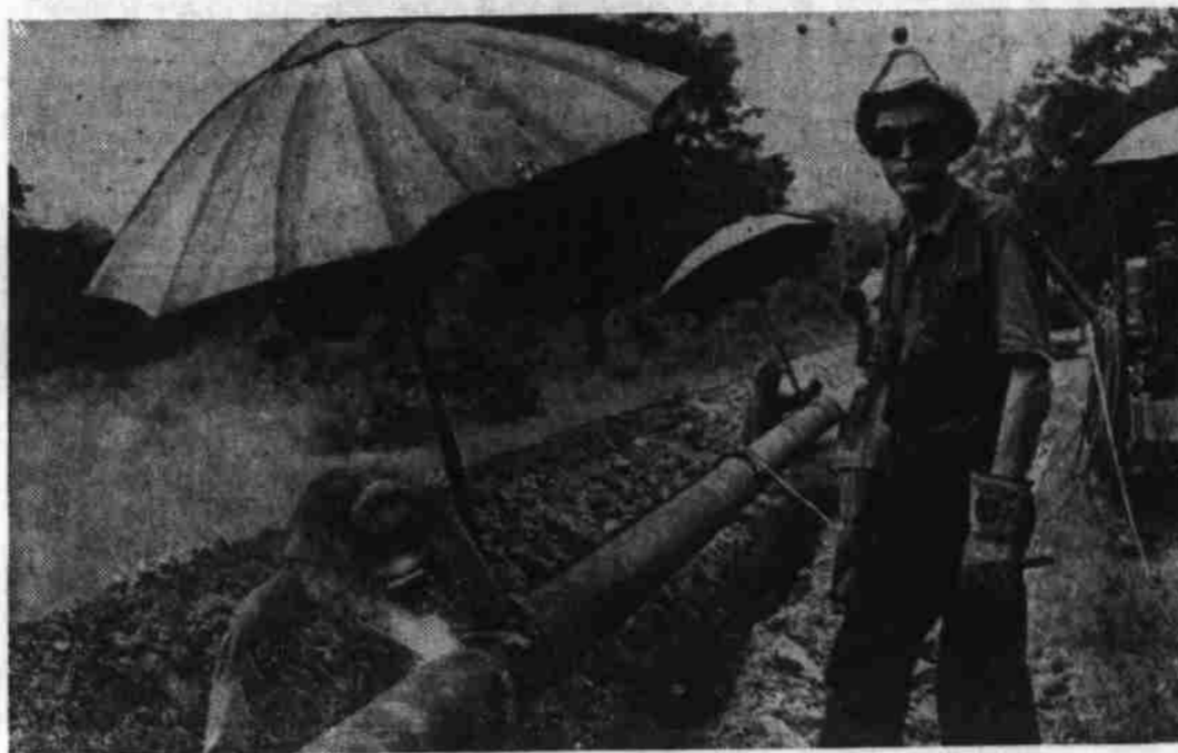
Because it is 99 in the shade not counting the heat from the arc, welders on the pipeline that is being rushed to feed the oil-starved eastern seaboard are given some relief by the sunshades. The men work in pairs, one at each end of a pipe section. This particular line is made up of partially used pipe-line systems which were dug up and relaid in directions that will accelerate the flow of oil to the Atlantic seaboard from the oil fields of the southwest. (Central Press)
