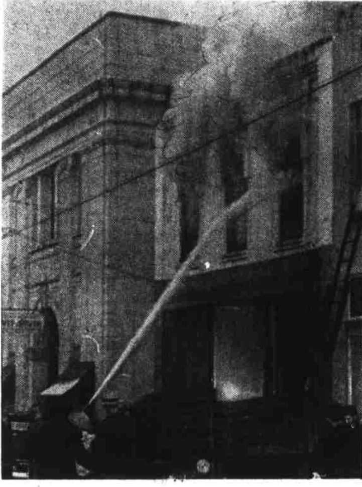
This photograph was made just as firemen started a stream of water into the second story of the Reeves Building on Main Street here last Wednesday afternoon. The building was damaged about $8,000. The vehicles parked along the street were moved within a few minutes after this picture was made by Jack Worthington of Skyland Studio.
